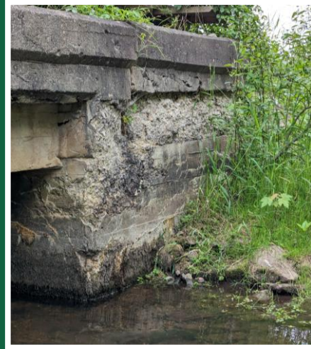
View of Deteriorated Abutment/wingwall
