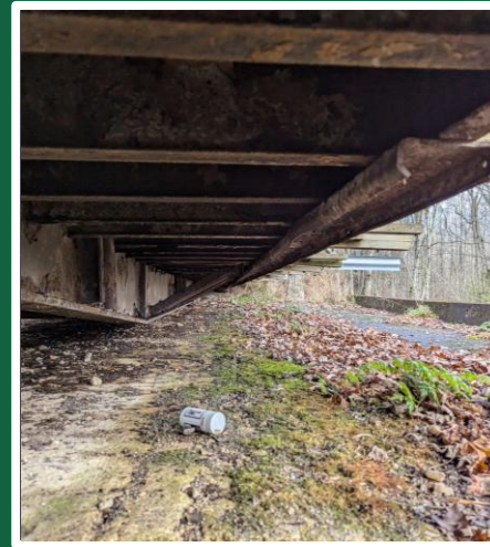
View of Superstructure Corrosion
