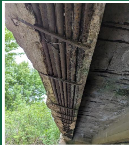
View of Exposed Rebar in Concrete T-Beam
