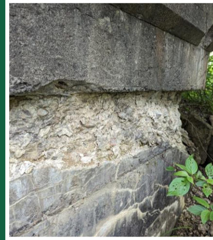
View of Wingwall Deterioration
