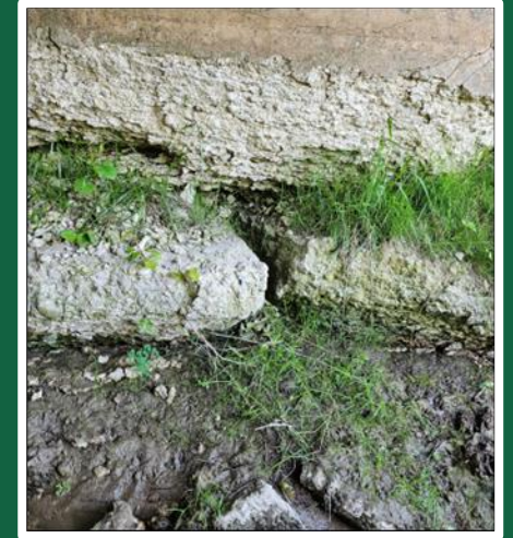
View of Wide Cracking at West Footing
