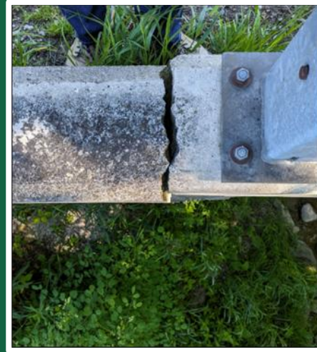
View of Wide Crack & Rotation at Wingwall
