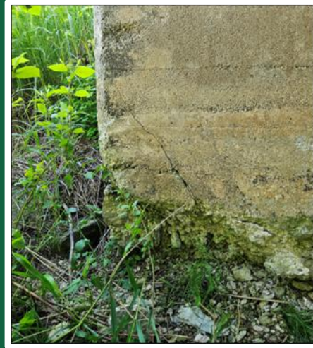
View of Spalling on East Abutment
