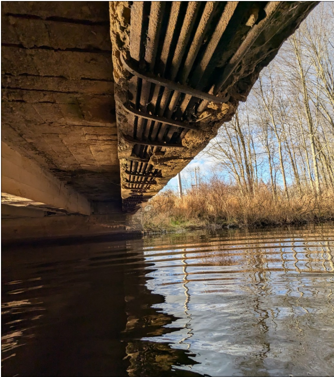
Photo 5 - View of Concrete Structure Girder Deterioration.
