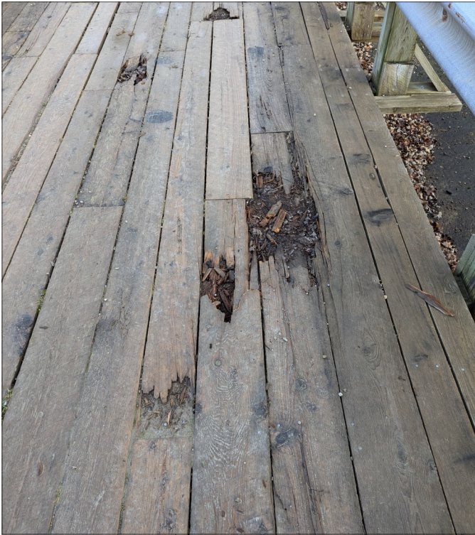
Photo 5 - View of Deteriorated Deck Boards.
