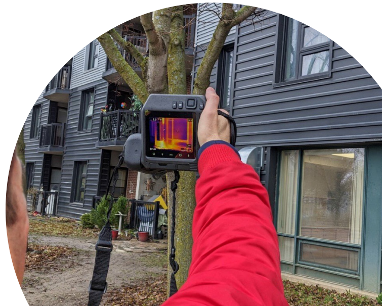
Infrared scanning of heat loss at Parkway Apartments
