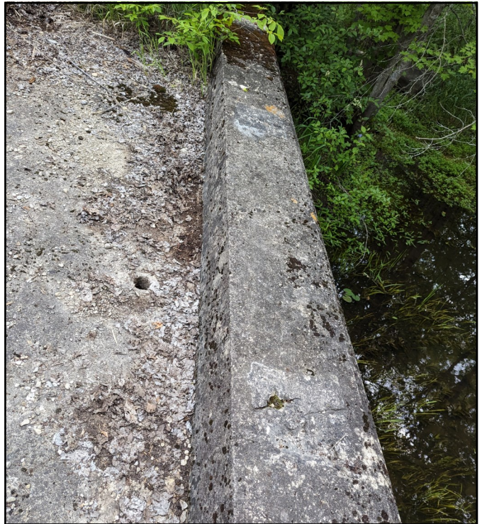
Photo 8 - View of Exposed Portion of Lower Structure Deck Top and Curb.
