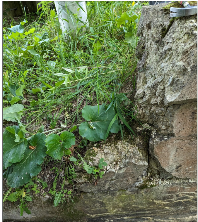
Photo 12 - View of Broken Section of Southeast Wingwall.
