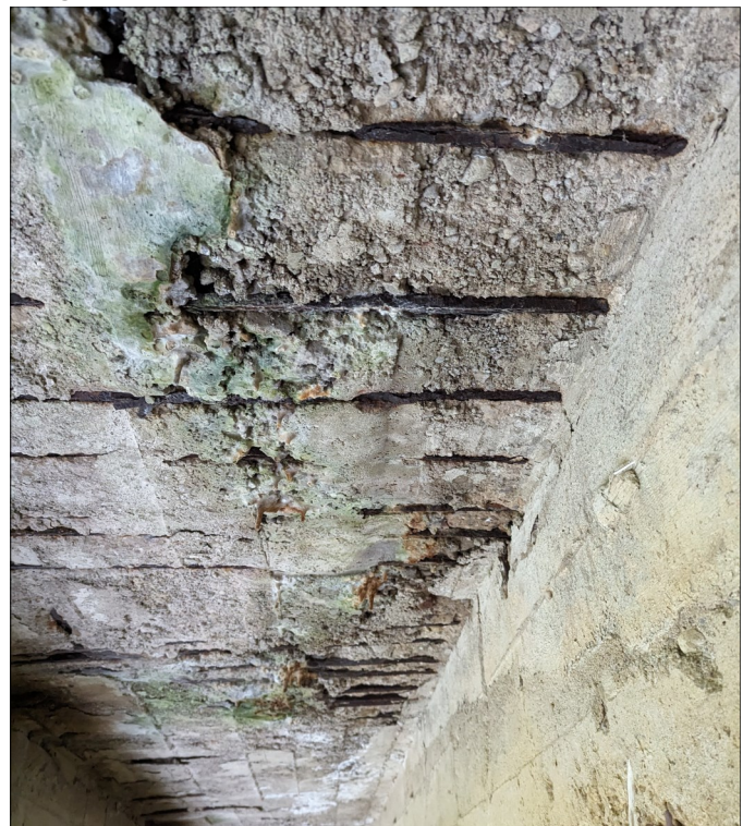
Photo 16 - View of Exposed Reinforcing at Interior Soffit.
