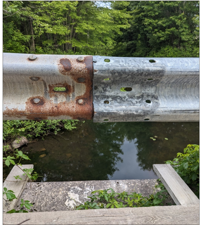
Photo 6 - View of Improper Barrier Lap Splice (typ.).
