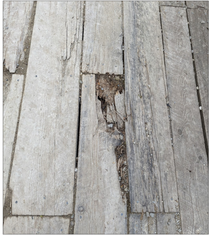
Photo 4 - View of Rotten Deck boards (typ.).
