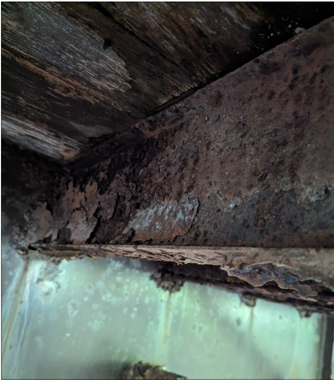
Photo 9 - View of Extensive Light to Medium Corrosion of Steel Stringers.
