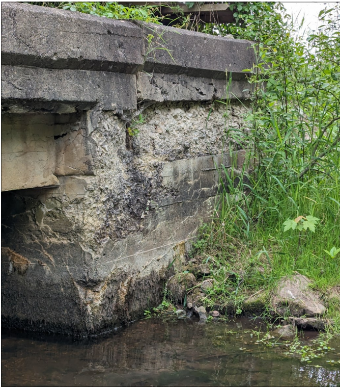
Photo 13 - View of Deteriorated Wingwall at Northeast.
