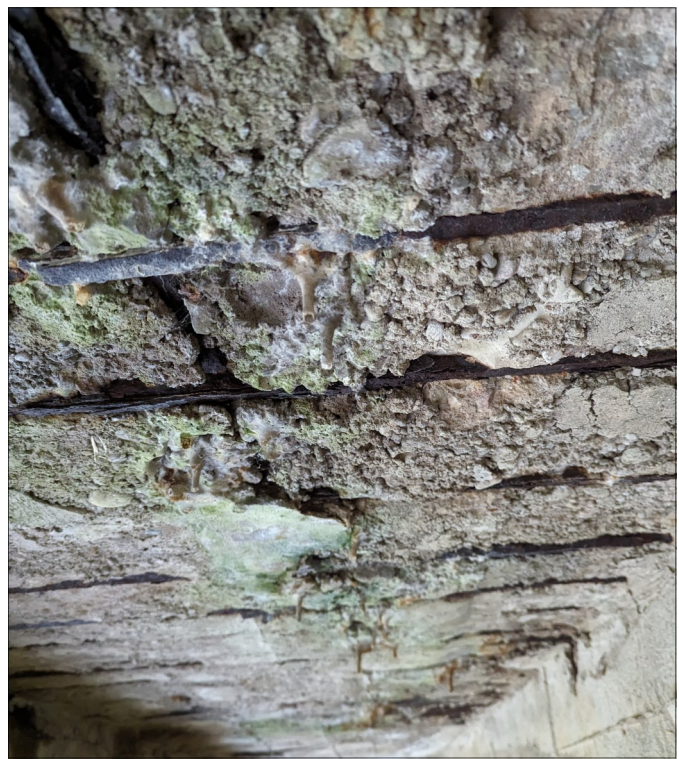
Photo 14 - Evidence of Water Penetration Through Original Deck Top.
