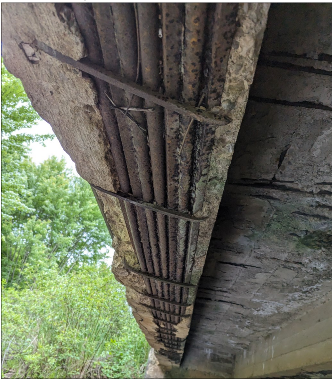
Photo 11 - View of Exposed Reinforcing Below Exterior Concrete Girder.
