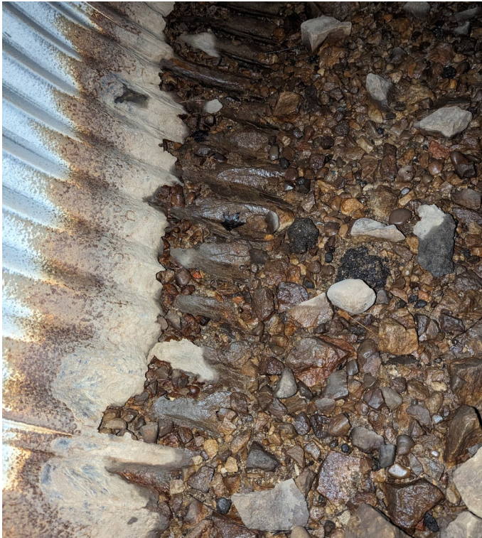
Photo 5 - View of Excessive Perforations at South Barrel Invert (Typ.)
