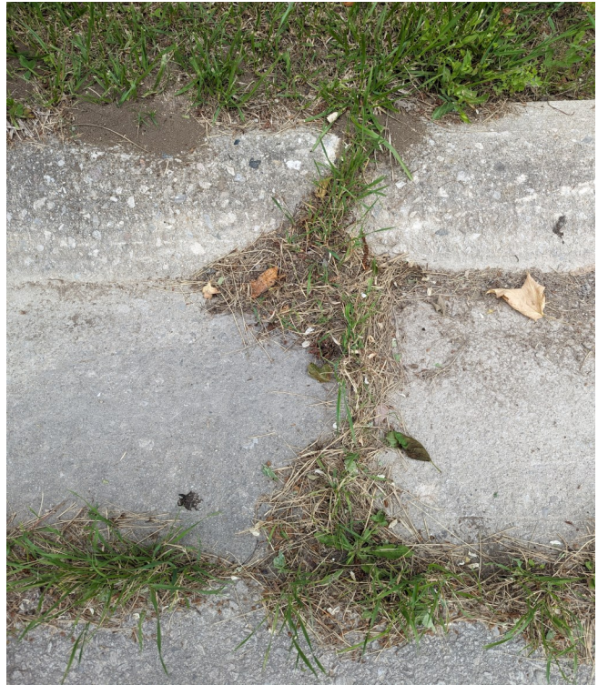
Photo 12 - View of Transverse Crack in Curb (Typ.)
