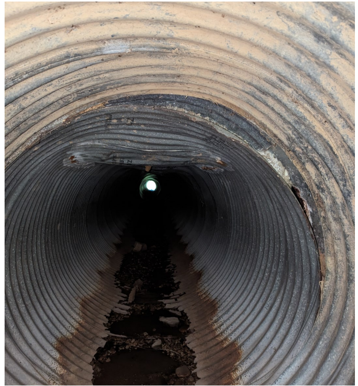
Photo 8 - View of Large Deformations at North Barrel Obvert (Typ.)
