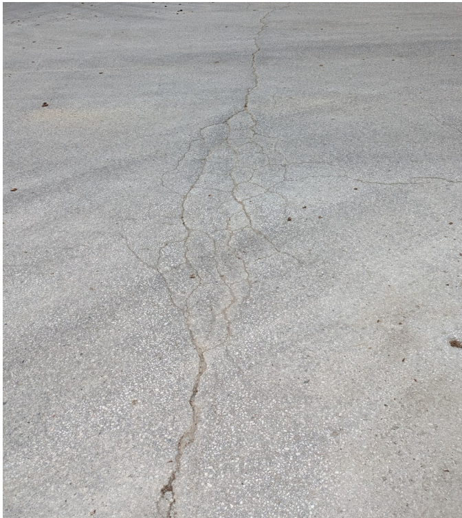
Photo 11 - View of Map Cracking in Wearing Surface Over Structure.
