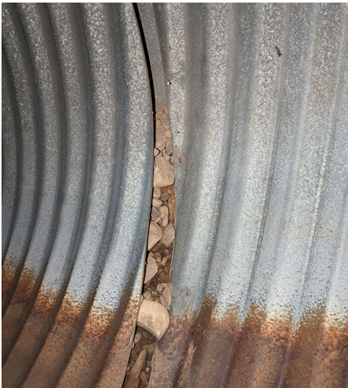
Photo 7 - View of Joint Separation at North Barrel (Typ.)
