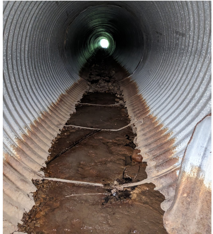
Photo 6 - View of Severe Section Loss at North Barrel Invert.
