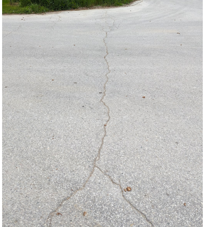
Photo 10 - View of Transverse Cracking in Wearing Surface Over Structure.
