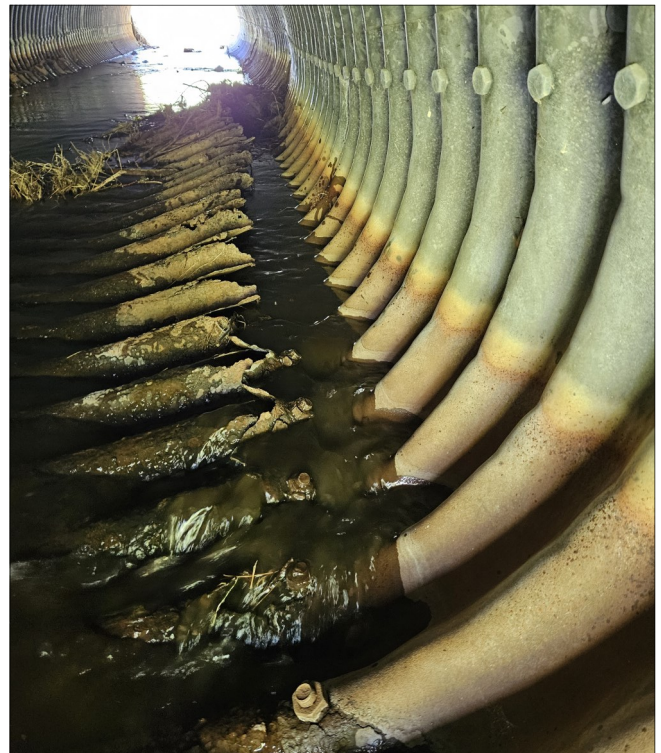
Photo 4 - View of Large Perforation on North Side of the Culvert.
