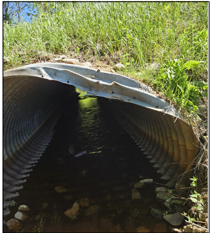
Photo 8 - View of Damaged Invert — West End.
