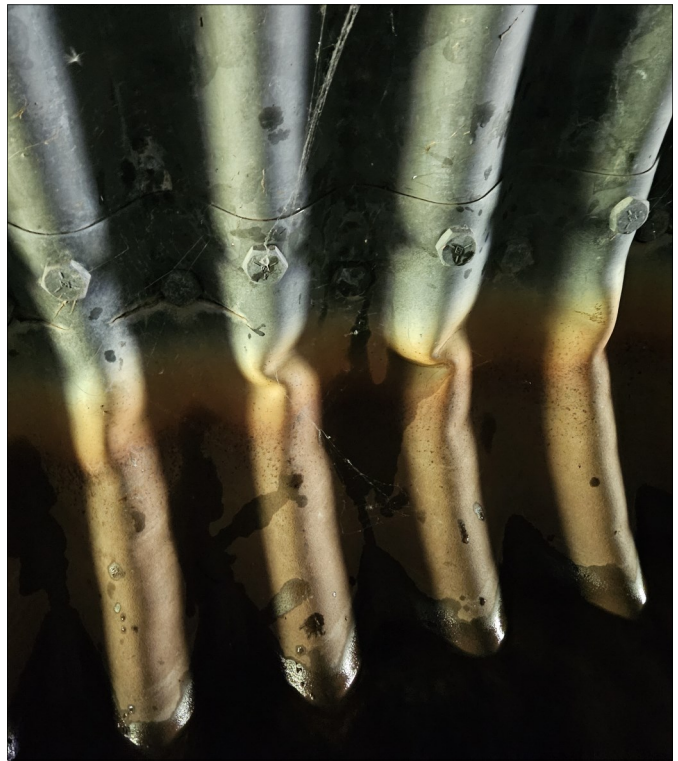
Photo 6 - View of Local Buckling of Corrugations North Side of Barrel.
