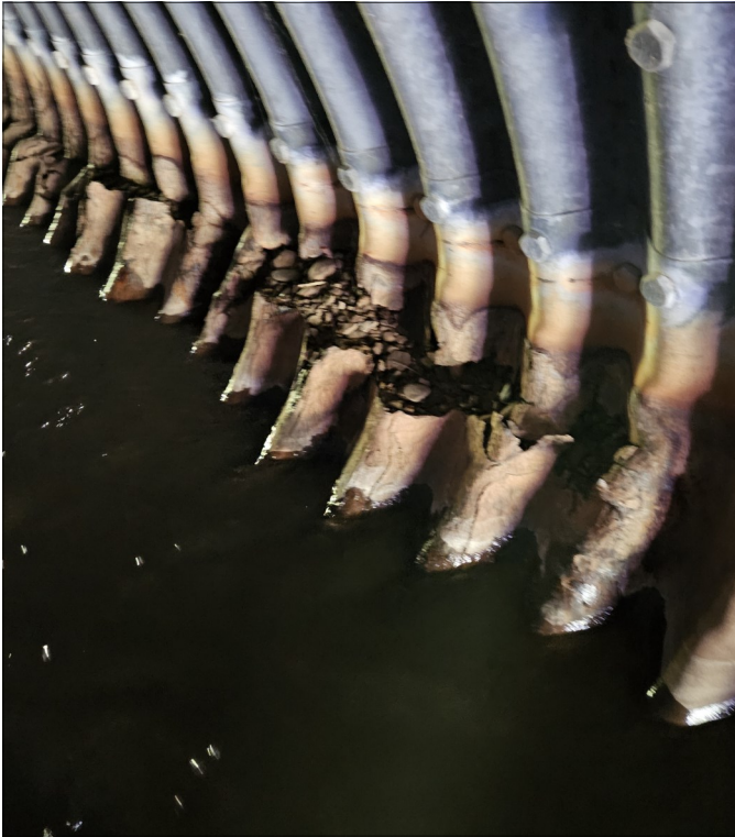
Photo 5 - View of Large Perforation on South Side of the Culvert.
